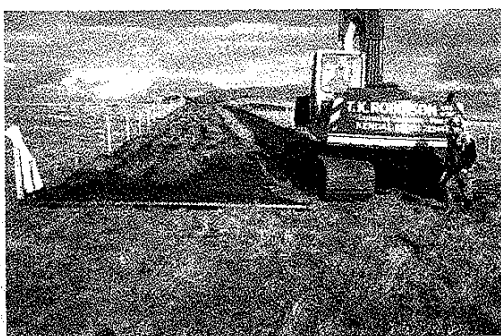
Plate 6.29 Turves being stored temporarily (no more than three weeks) on Crosby Ravensworth, Cumbria for a pipeline
